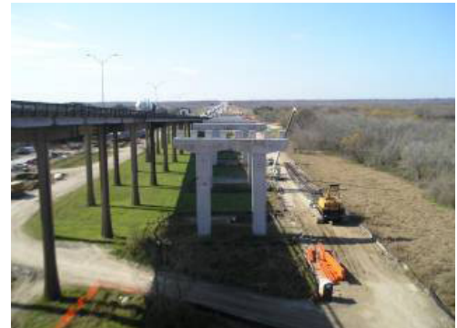
Trinity River Bridge, I-10 Near Houston, Texas. Provided Construction Engineering for balanced Cantilever Bridge.
